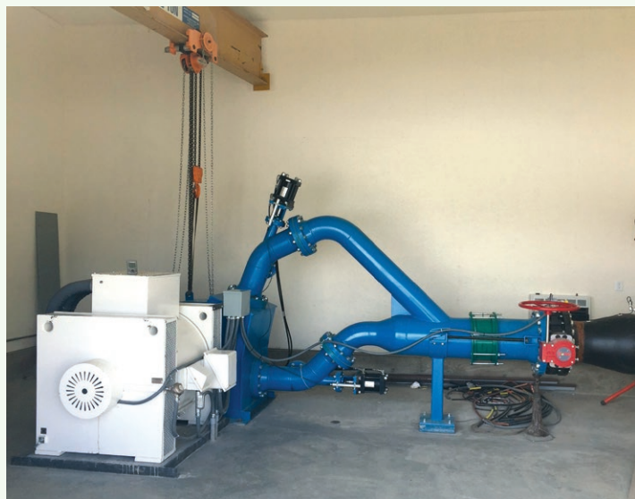
Fulton Hydropower Project turbine-generator unit (image courtesy of Gordon Fulton)
