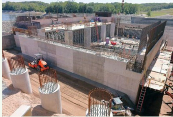
Red Rock Hydroelectric Project powerhouse overview during construction (image courtesy of Missouri River Energy Services)
